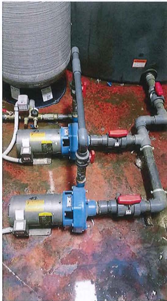
Dual Goulds 3656/3756 S-Group 1x2-8 Booster Pumps
