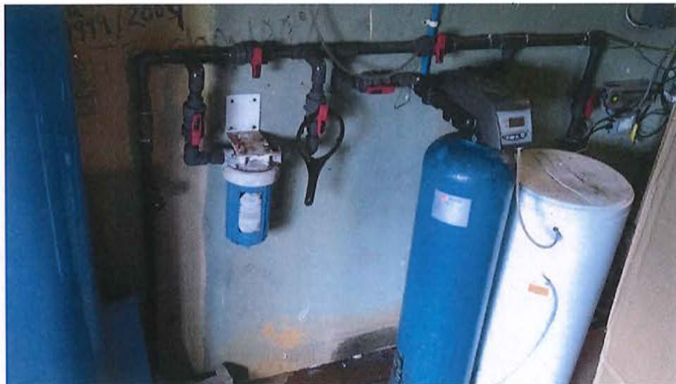
Second View of New Check Valve and Relocated Raw Water Tap
