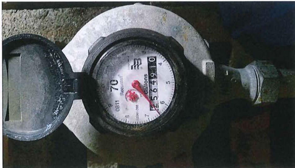
Water Meter Gauge
