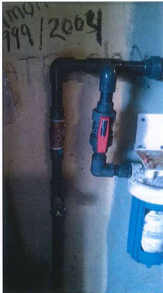
New Check Valve between Treatment and Relocated Raw Water Tap Installed in April 2015
