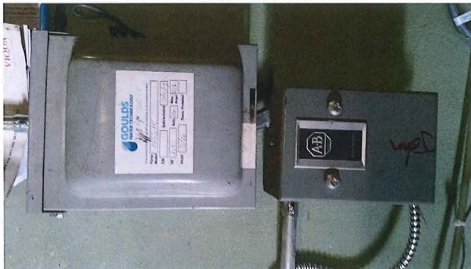
Supply Well Control Unit
