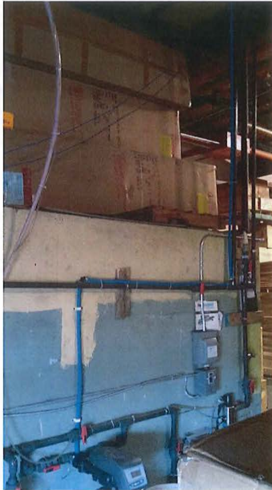
Revised Water Softener Backwash Discharge Pipe (Blue ¾" Pipe) Completed in April 2015
