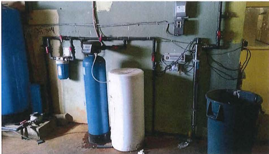
Second View of Water Treatment Components
