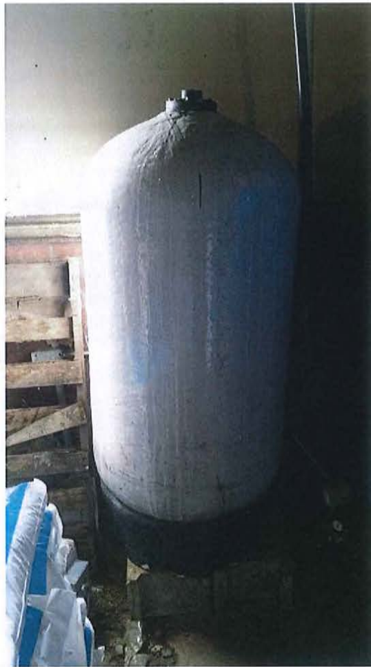
Existing Offline Pressure Tank
