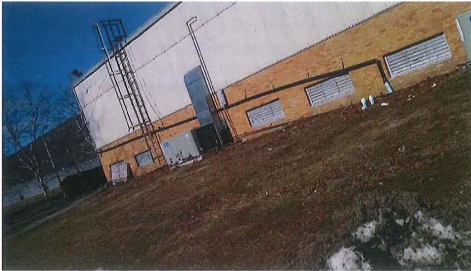
Water Softener Backwash Pipe connection to Existing Tile Field as of February 2015
