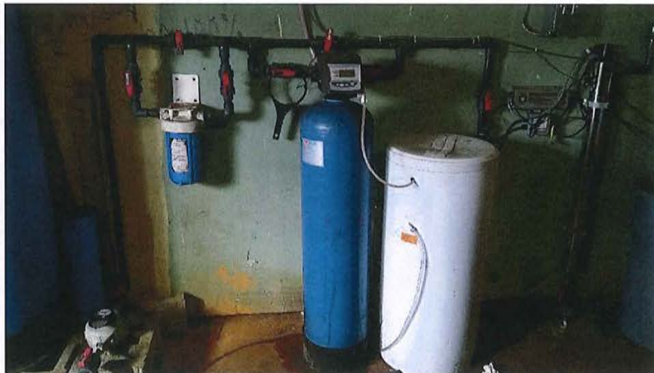
View of Water Treatment Components Including Aqua-Pure Water Filter, Master MP-MBA-60T-1 Water Softener, and Sterilight Platinum SPV-950 UV Treatment
