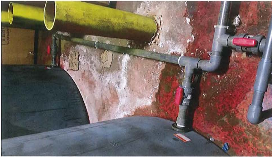
Piping Configuration for Poly Storage Tanks
