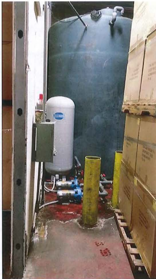
Water Storage Area Including Two 5,000 Gallon Poly Storage Tanks, Two Booster Pumps, Control Panel, and Water Pressure Tank
