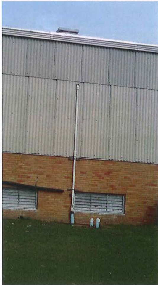
Revised Water Softener Backwash Discharge Pipe Connection to Existing Tile Field Completed in April 2015. Pipe was Rerouted Through Building to Avoid Future Breakage.
