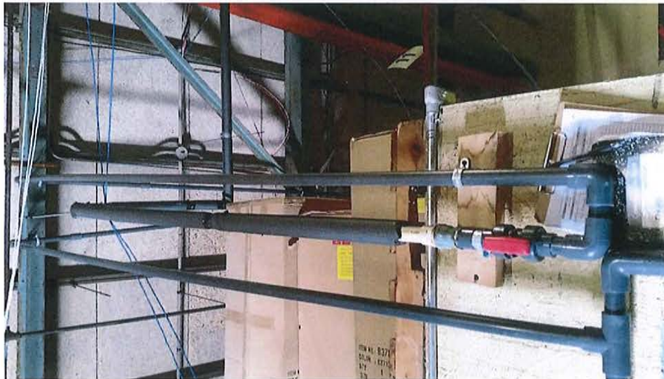
View of 1-1/4" PVC Piping To and From Storage
