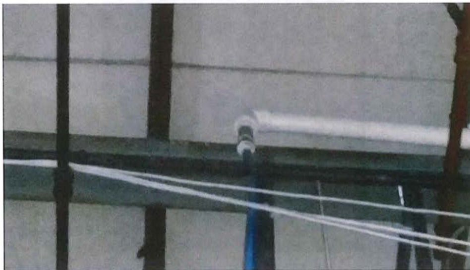
Revised Water Softener Backwash Discharge Pipe (Blue \frac{3}{4} " Pipe) Connection to 2" PVC Outlet Pipe Completed in April 2015
