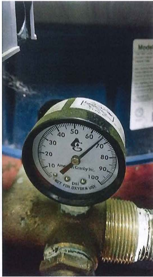
Pressure Gauge Reading at Flex-Lite FL40 Pressure Tank
