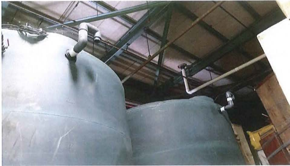
Emergency Overflow of Dual 5,000 Gallon Poly Storage Tanks
