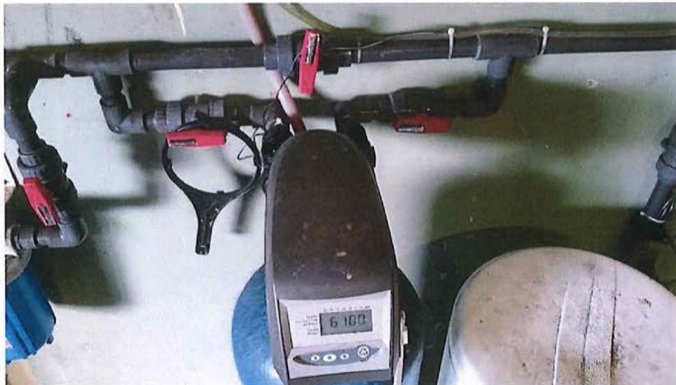
Water Softener Connection
