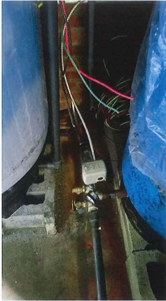
Pressure Switch, Gauge, and Drain Tap
