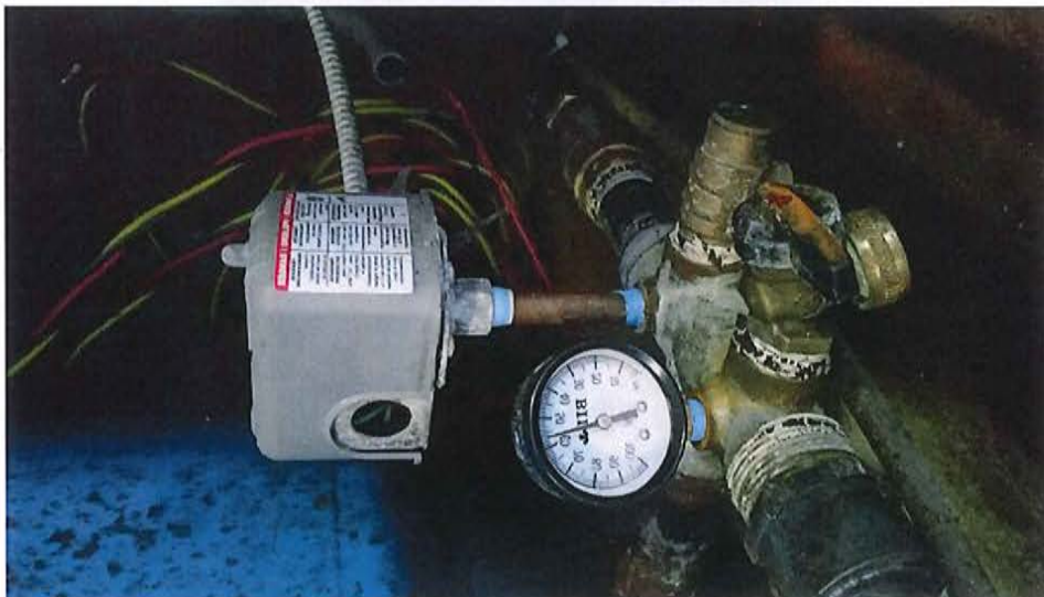
Pressure Switch, Gauge, and Drain Tap
