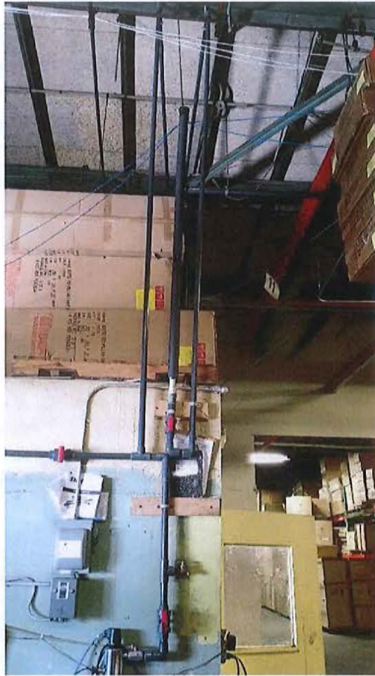
View of 1-1/4" PVC Piping To and From the Storage Tank Area and To the Distribution System
