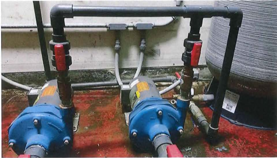
Dual Goulds 3656/3756 S-Group 1x2-8 Booster Pumps
