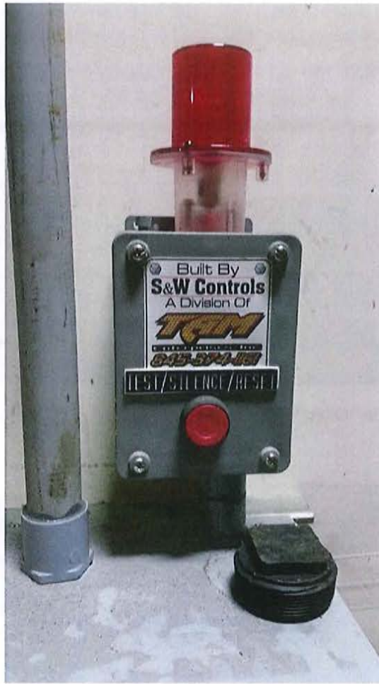
Control Panel Alarm
