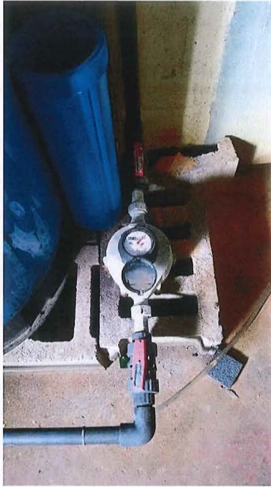
Water Meter Gauge Located Next to Dual Pressure Tanks
