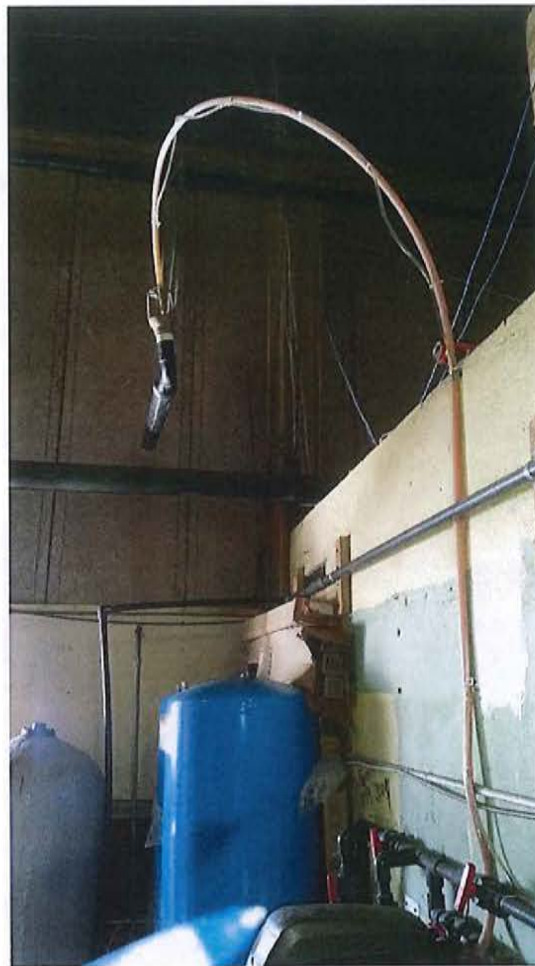
Water Softener Backwash Discharge Pipe as of February 2015
