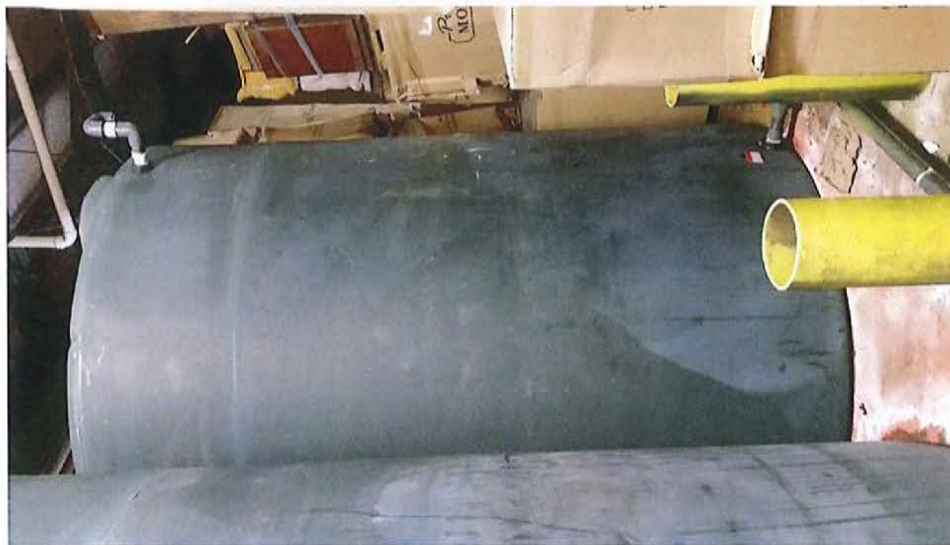
View of Side by Side 5,000 Poly Storage Tanks
