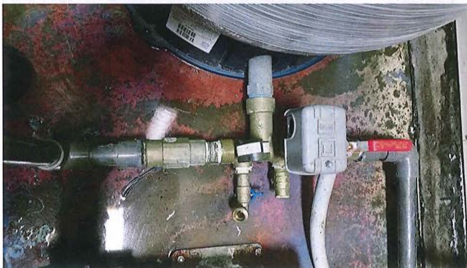
View of Check Valve, Pressure Switch, Pressure Gauge and Drain Tap at Flex-Lite FL40 Pressure Tank
