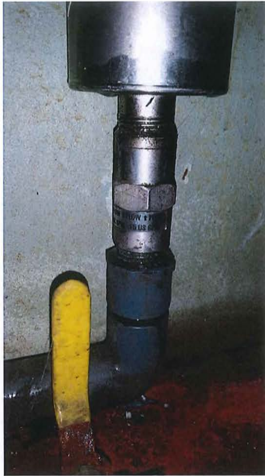
15 Gallon 9er Minute Flow Restrictor Located Below UV Treatment
