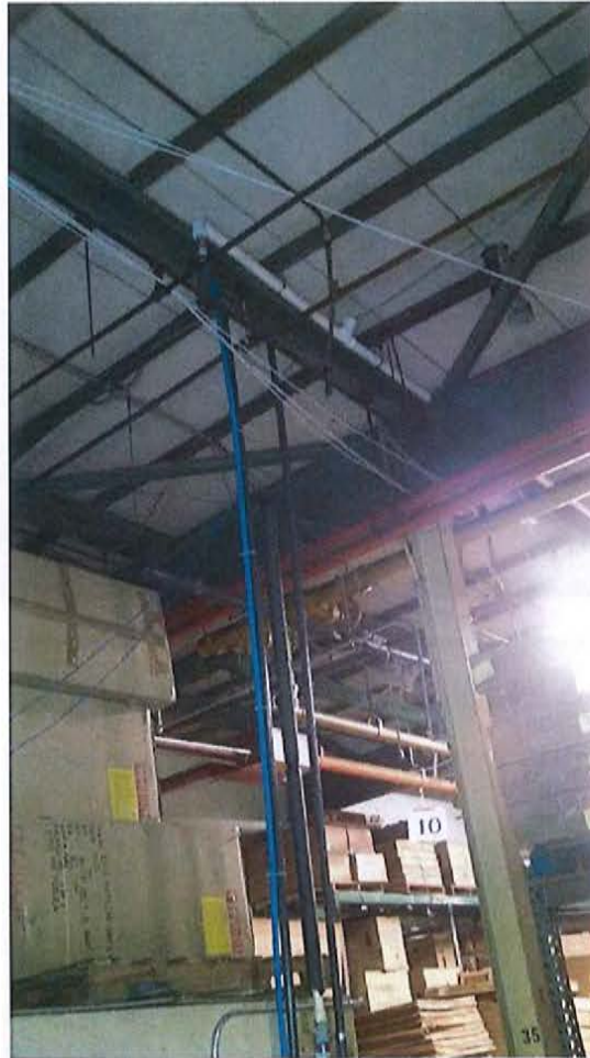
Revised Water Softener Backwash Discharge Pipe (Blue \frac{3}{4} " Pipe) Connection to 2" PVC Outlet Pipe Completed in April 2015
