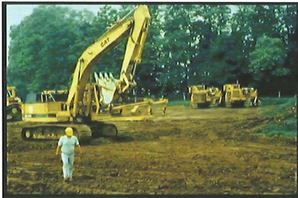
Fig. 14. The severely compacted soil of a temporary construction yard used daily by heavy equipment for four months; shown before deep ripping, topsoil replacement, and decompaction.
