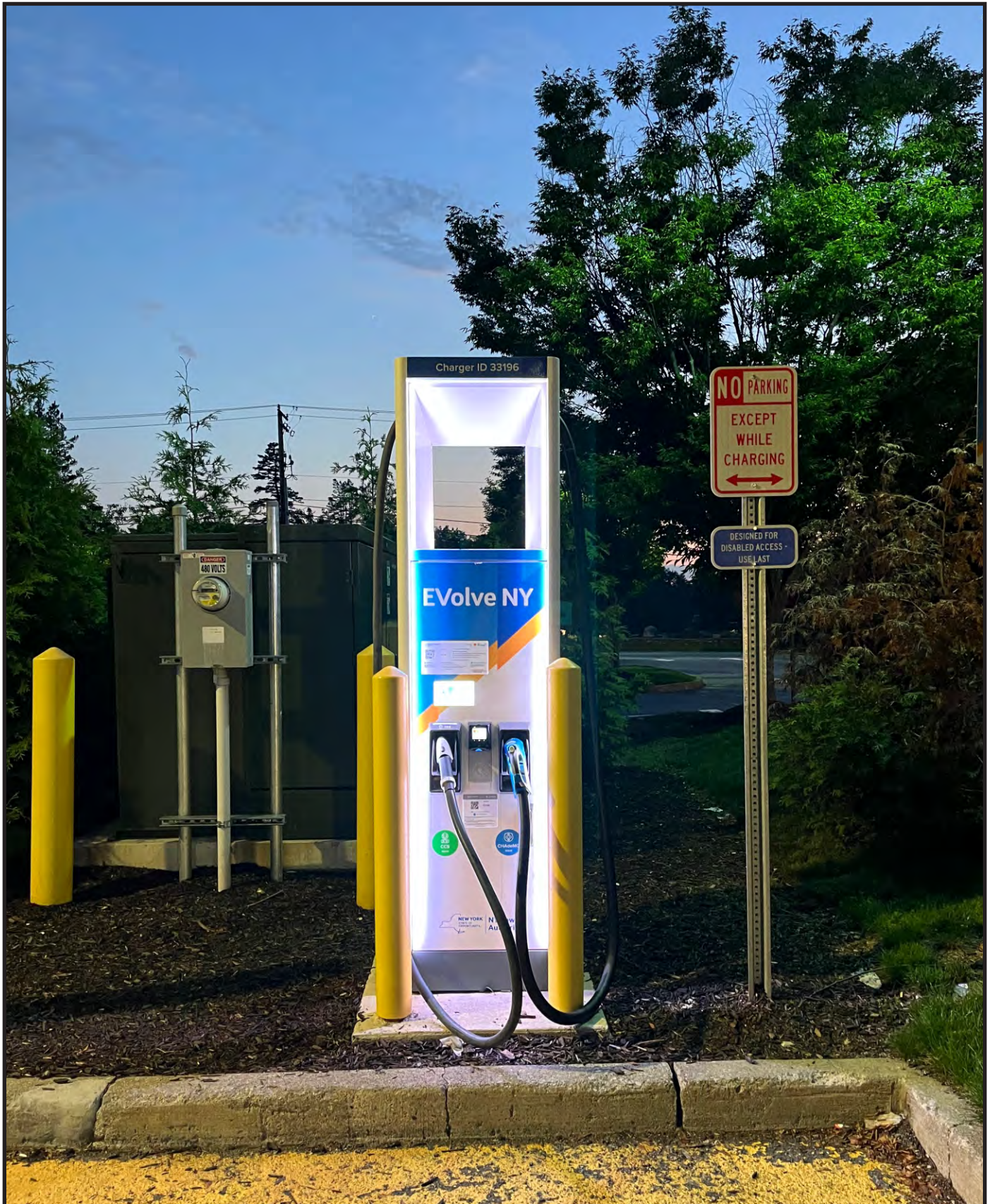
Figure 2-9: Example Electrical Vehicle Charging Station Monroe 208 Business Center Village of Monroe, Orange County, New York Source: TMA Photo
